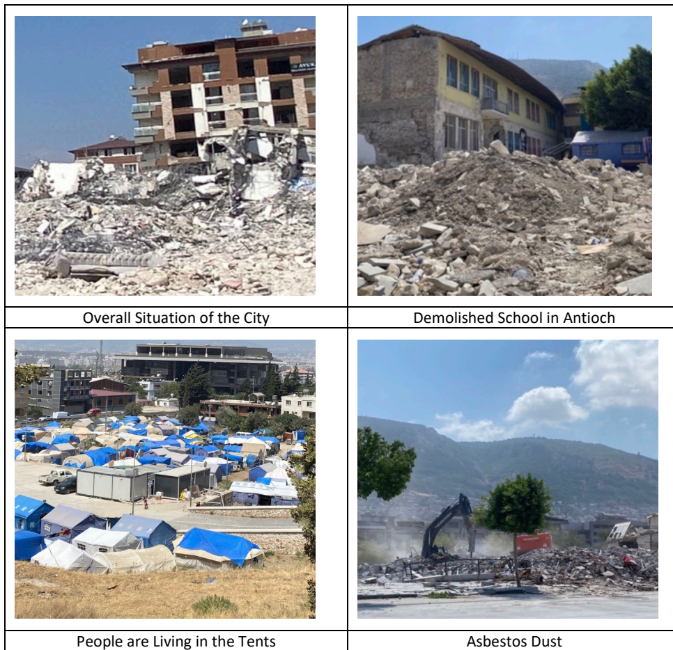
Figure 14 Post-earthquake situation of Antioch (Pictures taken by Kalkan, 2024)
