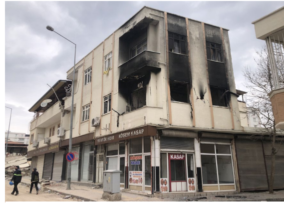
Figure 4b Fire following earthquake (photo from Nurdağı, Gaziantep).
