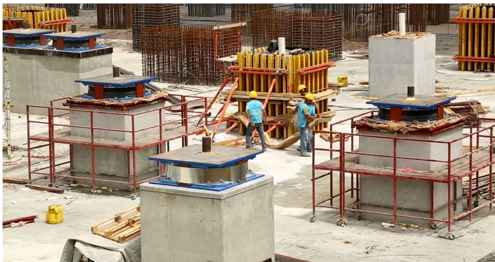
Figure 2 Göztepe Training and Research Hospital Construction Seismic Isolator Usage (İPKB, 2023)
