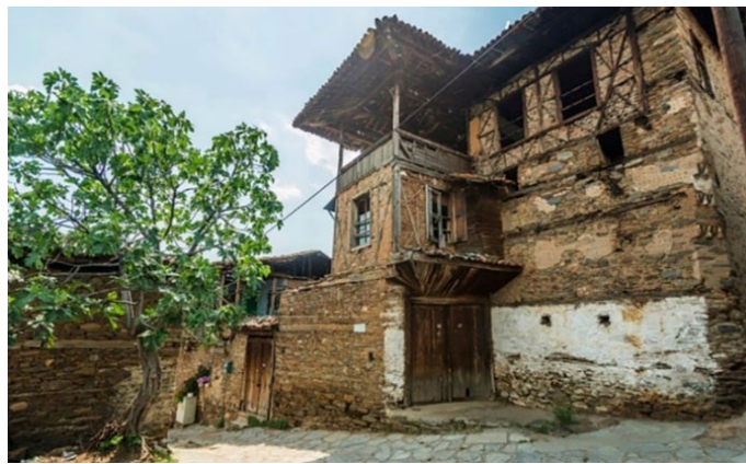
Figure 10 Abandoned traditional house, Birgi, İzmir (Küçük Oteller, 2018)
