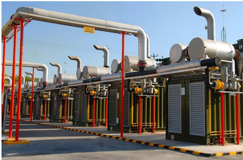
Figure 1 Monterrey Power Plant, Mexico ( https://www.sodensen.org.tr/ )
