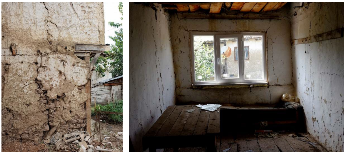
Figure 22 Damages in the buildings
