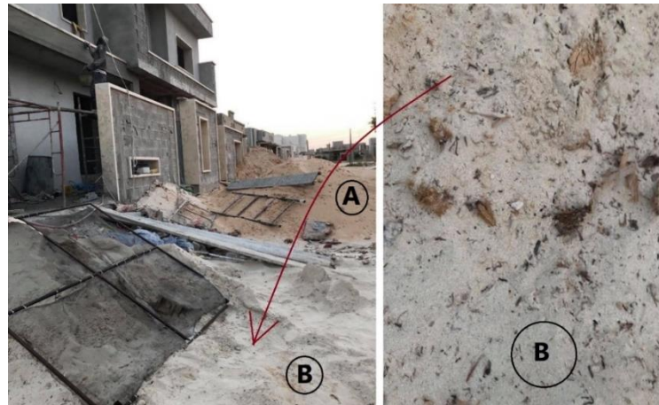
Figure 2 Photo taken by the researcher (2019) showing a building under construction using beach sand (B) alongside normal construction sand (A)
