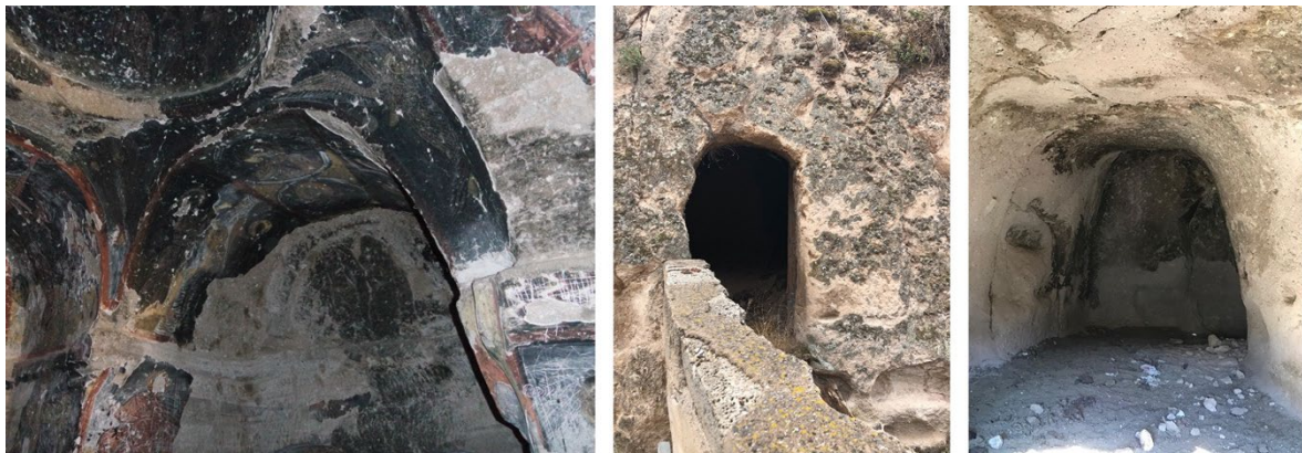
Figure 13 Various deterioration due to the natural and human-induced effects
