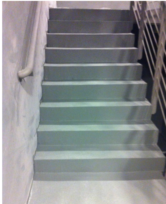
Figure 6 Example Fire Stair and Landing Epoxy Application (Parting sand surface epoxy) (Author Archive).
