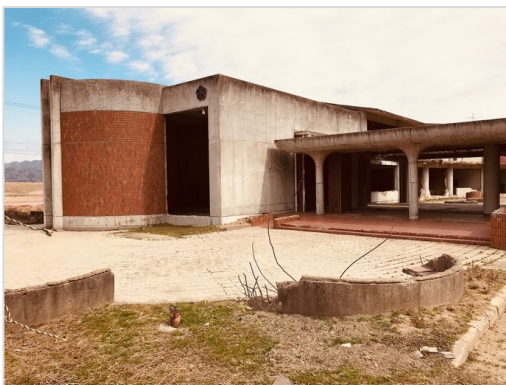
Figure 8 The earthquake-ravaged elementary school building in Miyagi Prefecture, Japan. (Photo by the Author)
